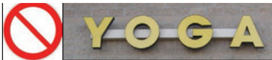
This exposed raceway would not be permitted because it is not integrated with sign design or colored to match the wall.
