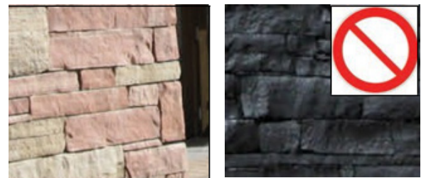
The color and striations of natural stone should not be compromised by staining or painting over the stone with a heavy coating
