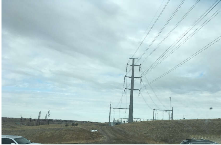
Description: Adjacent electrical substation View Direction: North
