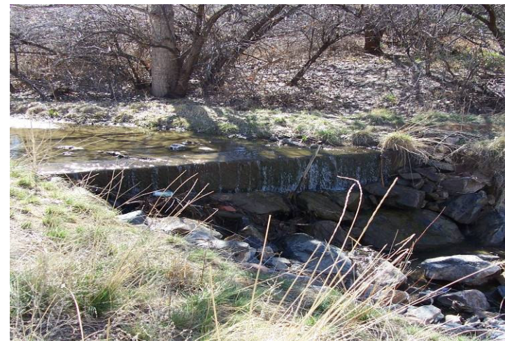
FIGURE 4-2 Exposed utility crossing on Greenwood Gulch
