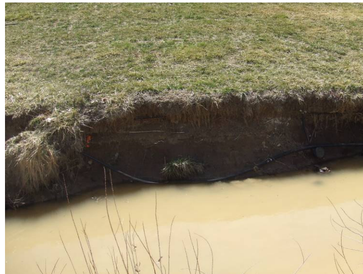
FIGURE 4-6 Low flow channel degradation, Little Dry Creek
