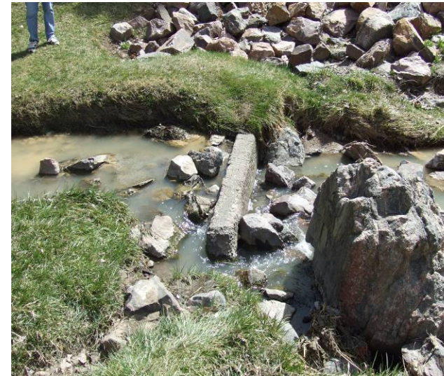
FIGURE 4-7 Failed check structure upstream of Arapahoe Road, Little Dry Creek
