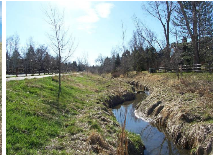
FIGURE 4-4 Greenwood Gulch portion of channel lacking capacity next to Orchard Drive
