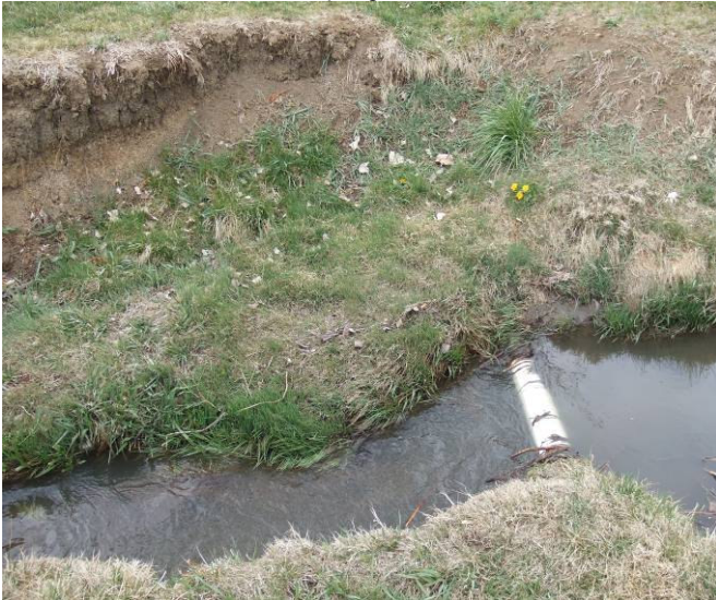
FIGURE 4-11 Low flow channel erosion on Spring Creek
