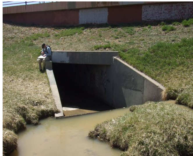
FIGURE 4-5 Undersized culvert crossing at Quebec Street on Little Dry Creek
