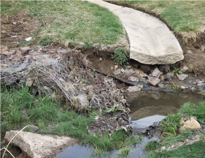
FIGURE 4-12 Channel erosion on Willow Creek
