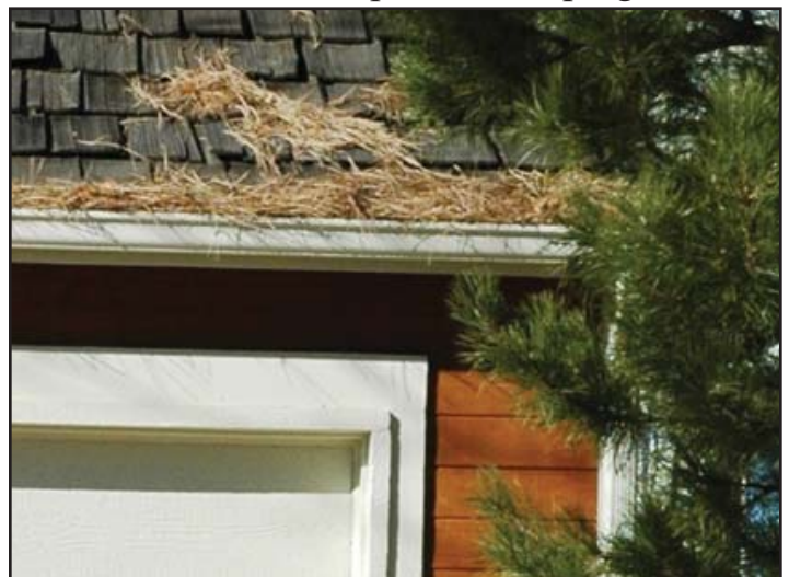
This roof is extra vulnerable to embers because needles have accumulated in the gutter below an aging wood-shake shingle roofing assembly. Photo by South Metro Fire Rescue.
