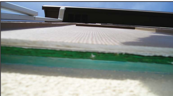
A gap between siding and the foundation at the base of a wall. Photo by Colorado Springs Fire Department.
