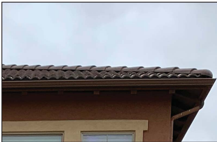
Although these roof tiles are curved, architects and builders were careful to form the layer below to prevent airborne embers from slipping under the tiles. Photo by South Metro Fire Rescue.
