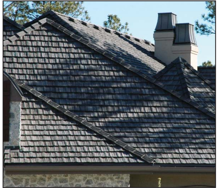
From a distance, this roofing looks like wood shingles, but it actually features tile shingles. It is a Class A fire-rated assembly. Photo by South Metro Fire Rescue.
