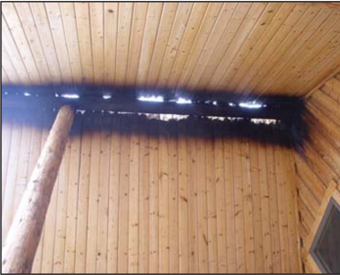
Damage to this wood home was limited to the ridge line, but screening the ridge vent could have prevented that damage. Photo courtesy of Rick Trenbath.
