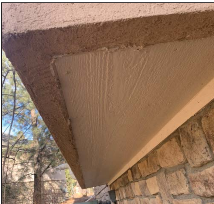
This projection is less vulnerable to pooling convective heat because it is protected by a layer of wood. Photo by South Metro Fire Rescue.
