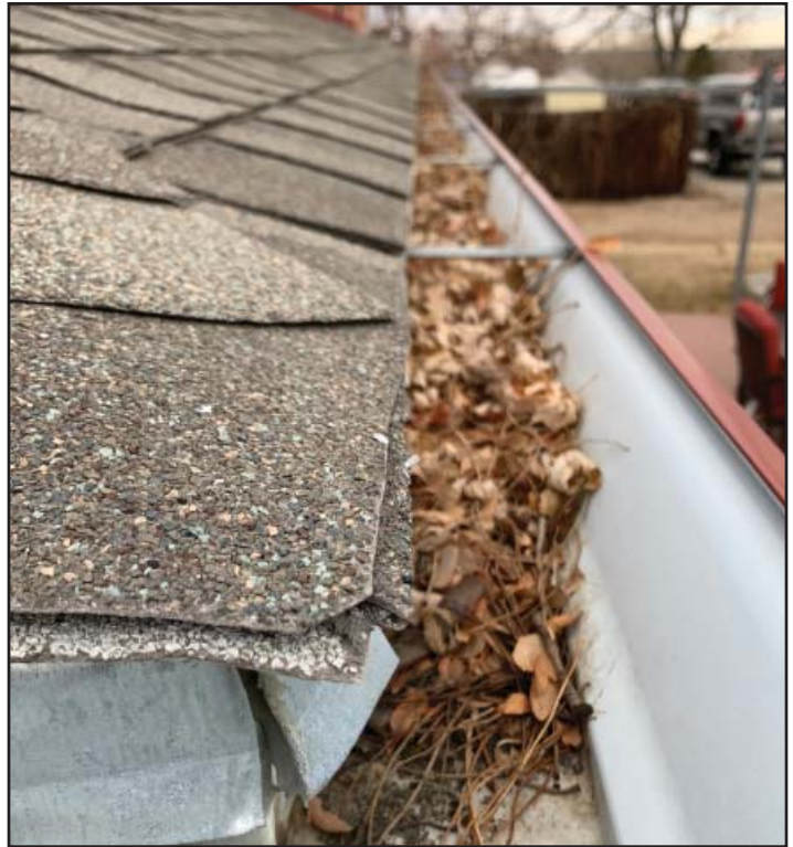
If these dead leaves catch fire, heat may flow under the asphalt shingles igniting the roof assembly and attic. A screen, such as one in the photo at right, prevents combustible debris from accumulating in gutters. Photos by South Metro Fire Rescue.
