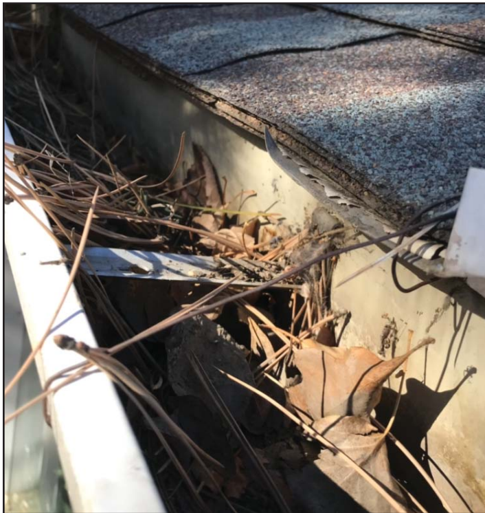
Dead needles and leaves in this gutter are easy fuel for spot fires caused by embers. Photo by South Metro Fire Rescue.
