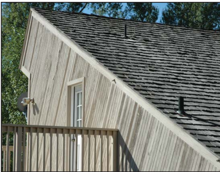
This unrated wood-shingle roofing assembly poses a significant hazard to its owners and residents downwind if the roof ignites. Photo by South Metro Fire Rescue.
