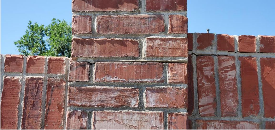
Figure 27. Example of Column Pop-Up distress with the cap buckling slightly higher on the right side.
