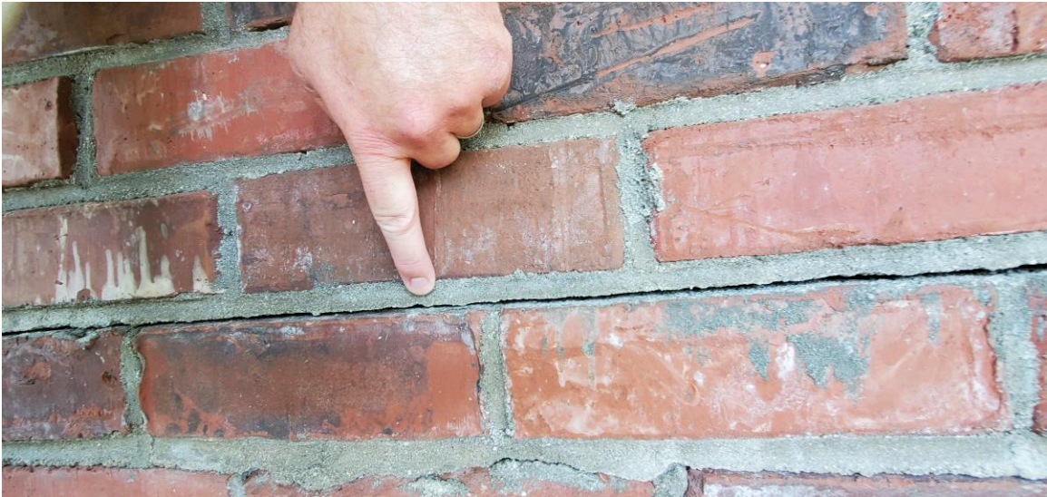
Figure 21. Example of "Sag Panel Sagging" distress, the moderate category of panel sagging.
