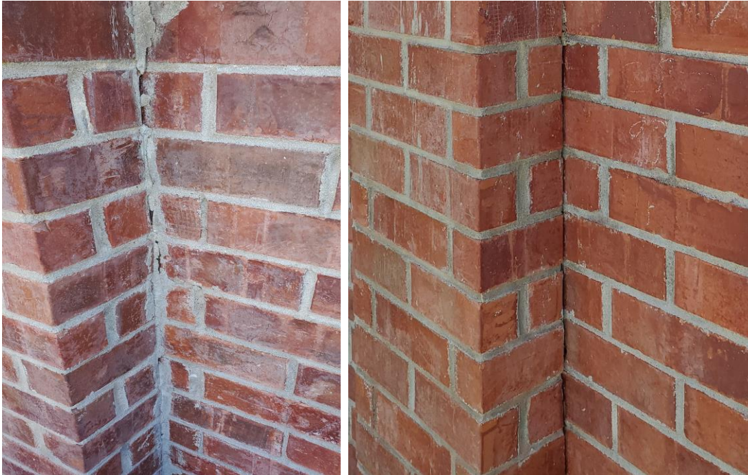
Figure 36 On the left is a panel solid expansion joint, and the photograph on the right shows a properly constructed panel expansion joint.
