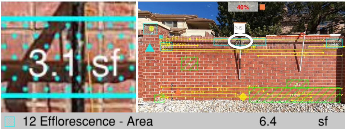
Figure 53. Efflorescence is represented by a stippled blue box and can be found anywhere on the panel or column. It is measured in square feet of area, and each panel can have multiple markings for efflorescence. In the legend, the value is displayed as the total area in square feet for all efflorescence areas.
