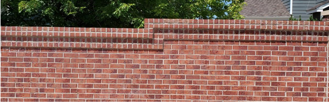
Figure 41. An example of a cap with less than 30% spalled units.
