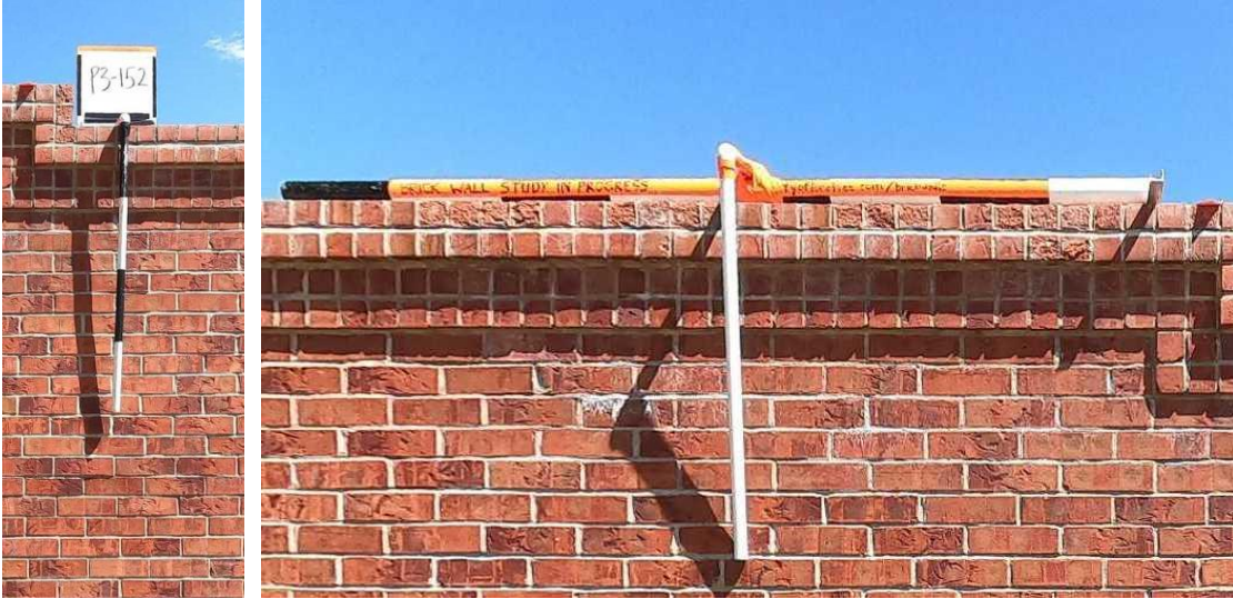
Figure 10. (Left) Whiteboard with panel number and vertical scale. (Right) Story pole striped to provide horizontal scale.
