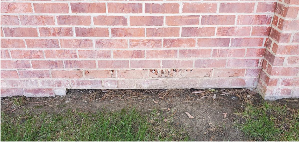
Figure 33. An example of panel spalling distress, likely related to retained soil on the opposite side of the wall.
