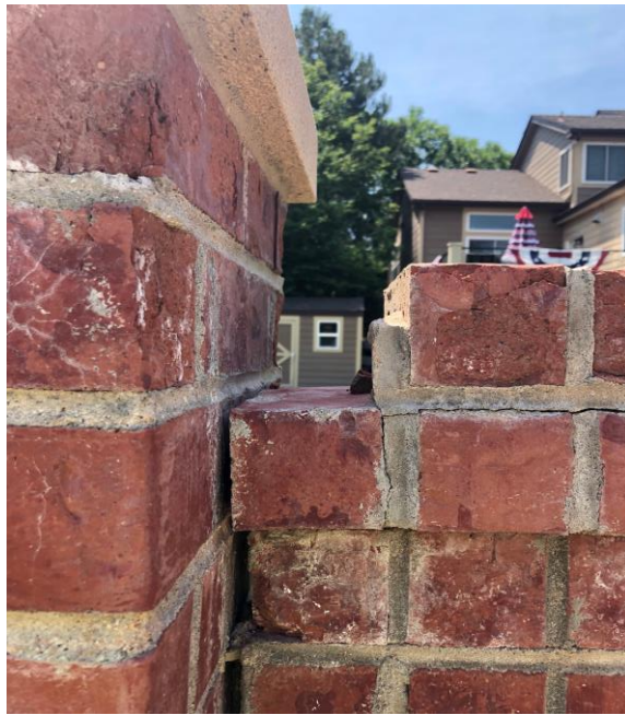
Figure 30. Example of a missing brick unit at a wall cap.
