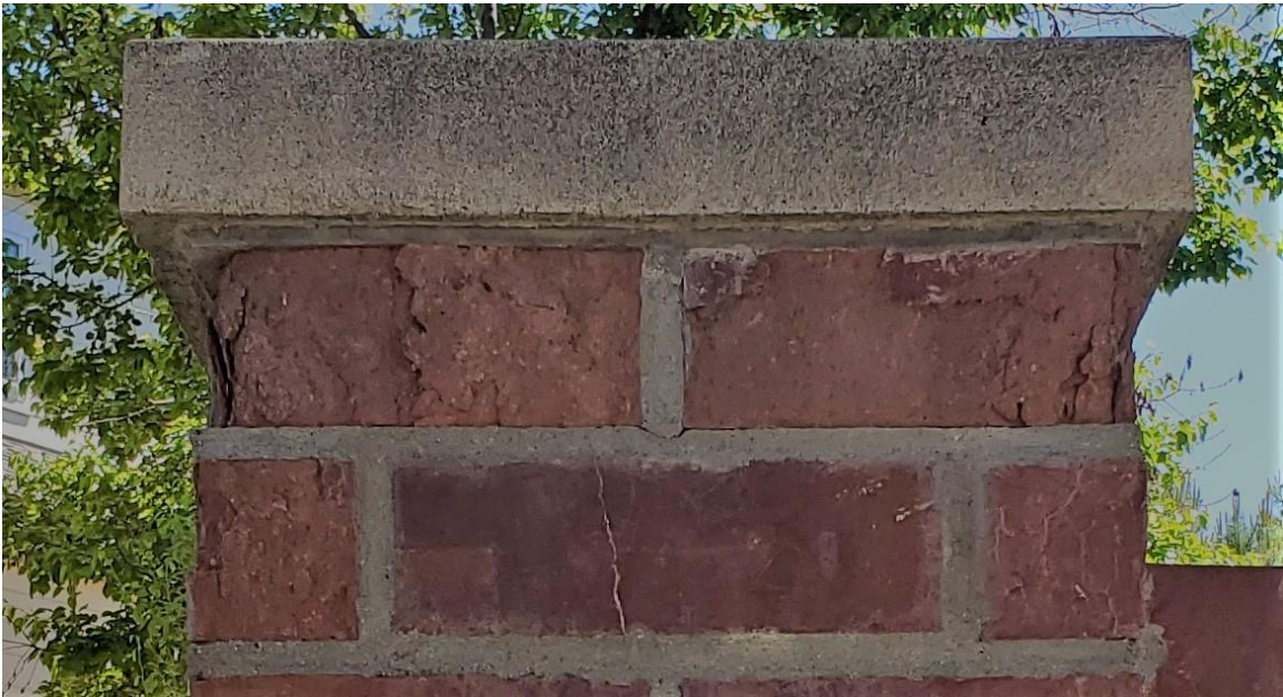
Figure 34. An example of brick spalling beneath a column cap.
