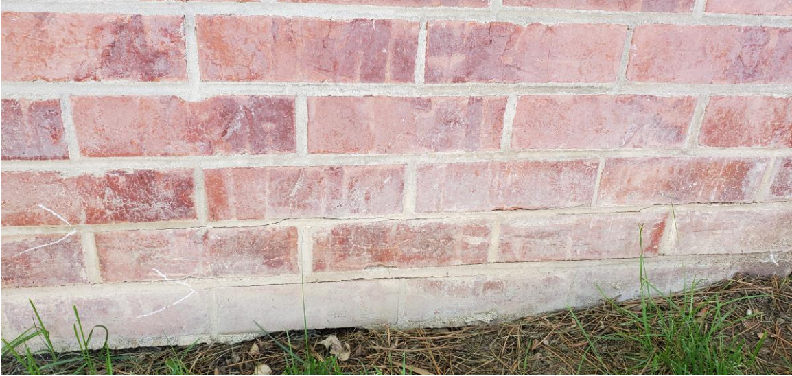
Figure 20. Example of "Crack Panel Sagging" distress, the minor category of panel sagging.
