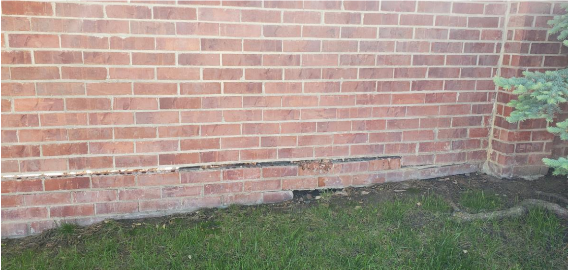
Figure 22. Example of "Collapse Panel Sagging" distress, the severe category of panel sagging.
