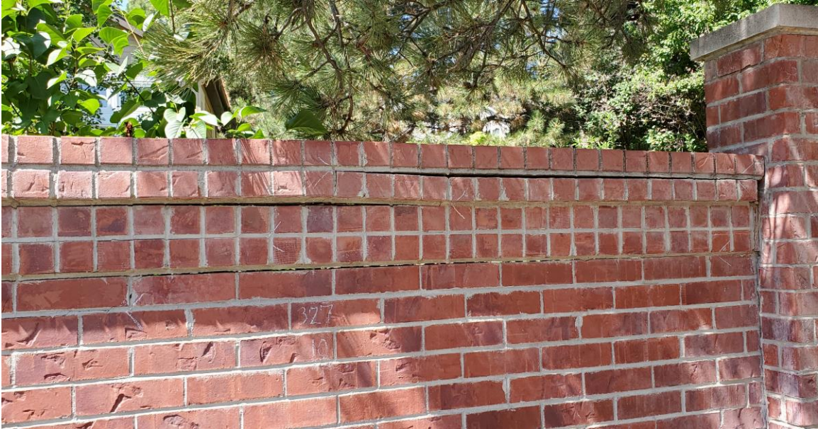
Figure 32. An example of horizontal cracking in and near a cap that is buckling due to expansion that is not accommodated with an open joint at the level of the cap.
