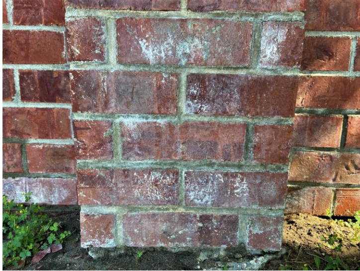
Figure 37. An example of efflorescence at a column.
