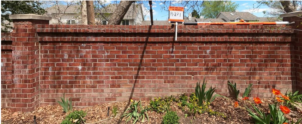
Figure 39. An example of a panel with significant retained soil viewed from the yard side. Approximately 15 courses of brick are visible in the panel above grade.
