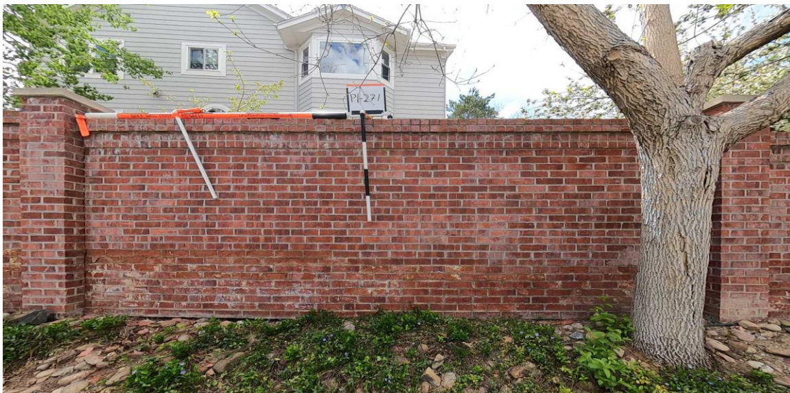
Figure 40. An example of a panel with significant retained soil viewed from the street side. Approximately 23 courses of brick are visible in the panel above grade (i.e. the soil on the back side is approximately 8 courses or 2 feet higher than the front).
