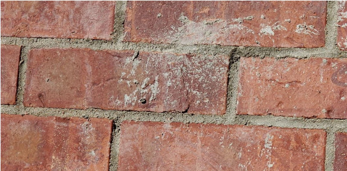
Figure 38. An example of mortar staining that was marked by ANA as an area for cleaning.
