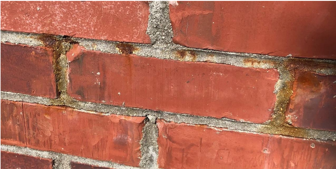
Figure 28. An example of corroding bed joint reinforcing.
