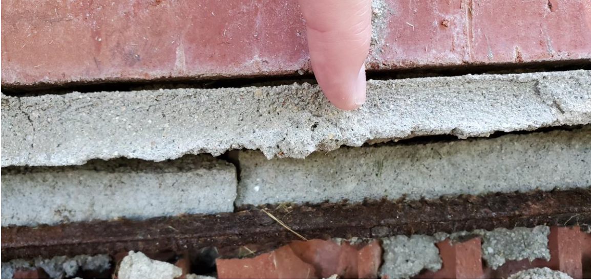
Figure 29. Example of corroded reinforcing bar in bond beam at the bottom of a panel.
