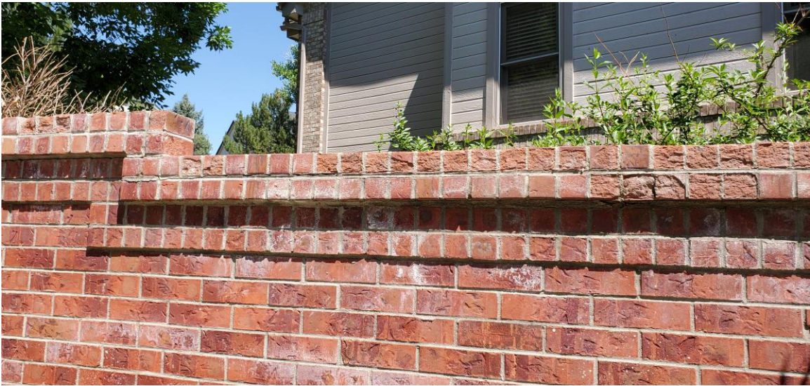
Figure 42. An example of a cap with 40% to 70% spalled units.
