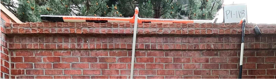
Figure 43. An example of a cap with 80% to 100% spalled units.
